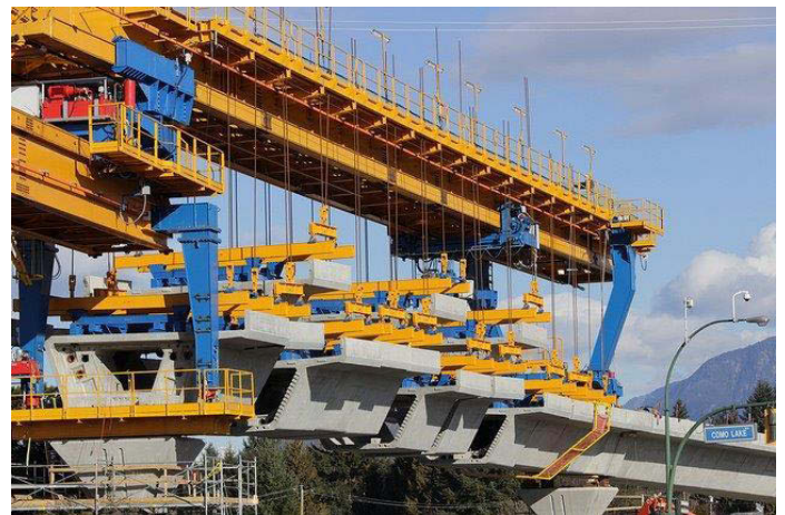
Photograph of the construction of an elevated guideway in the Burquitlam area.
