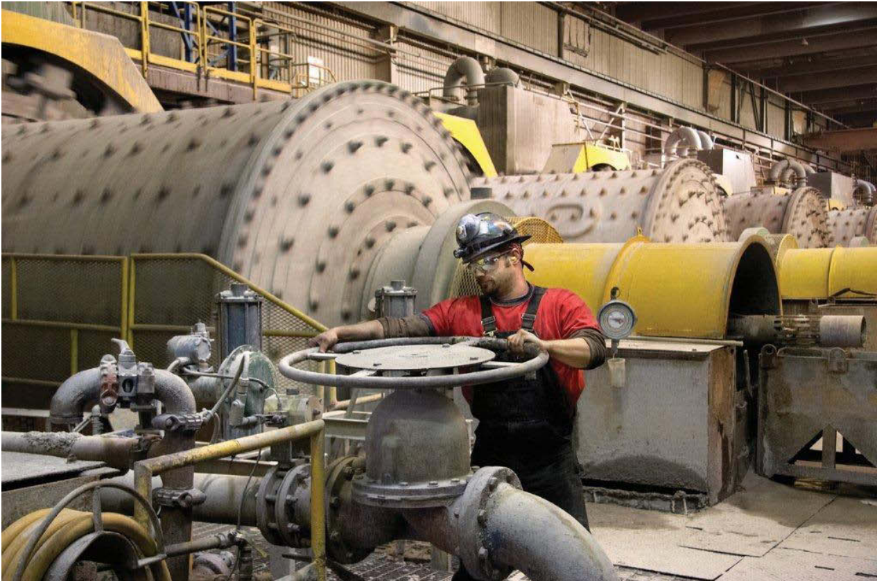
Inside the mill at Endako Mines, northwest of Prince George. An expansion of the mill was commissioned in the summer of 2012, and along with other upgrades to the molybdenum mine, will nearly double the ore processing capacity to 55,000 tonnes daily. The mine employs 420 skilled and professional workers.
