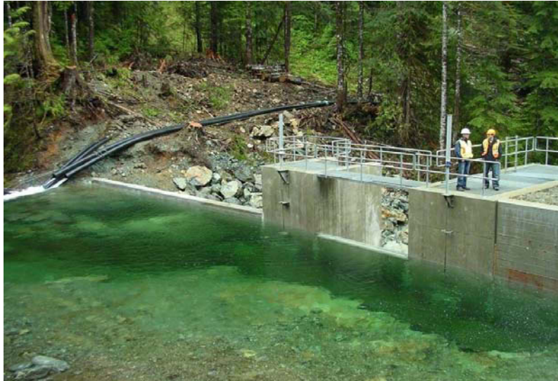
Canoe Creek Hydro on the Tla-o-qui-aht First Nation's traditional territory on Vancouver Island is a run-of-the-river hydropower project that generates clean electricity.
