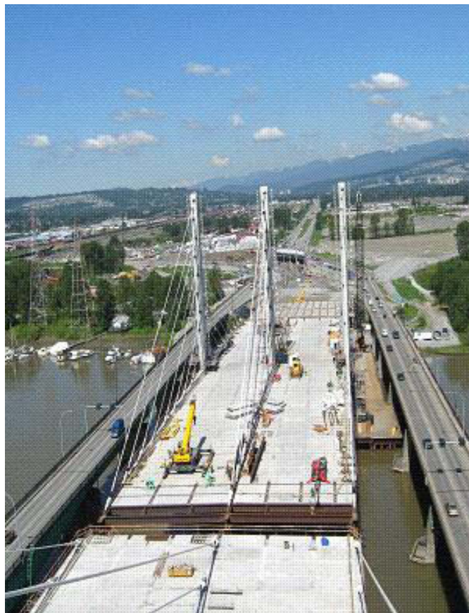
Pitt River Bridge westbound, May 2009, shows placement of deck panels is almost complete.
