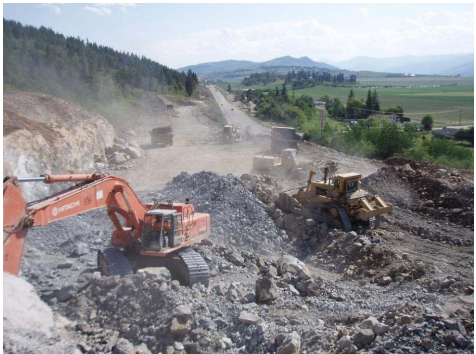
Okanagan Corridor - Excavator pulling material from a blast in the Larkin to Crozier segment. In the background, the existing Highway 97A remains open to the travelling public while the new four lane section of the highway is being constructed.
