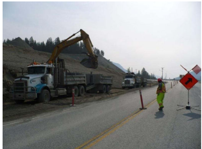
Construction of the fourth lane of Phase 3 West utilizing local hired equipment
