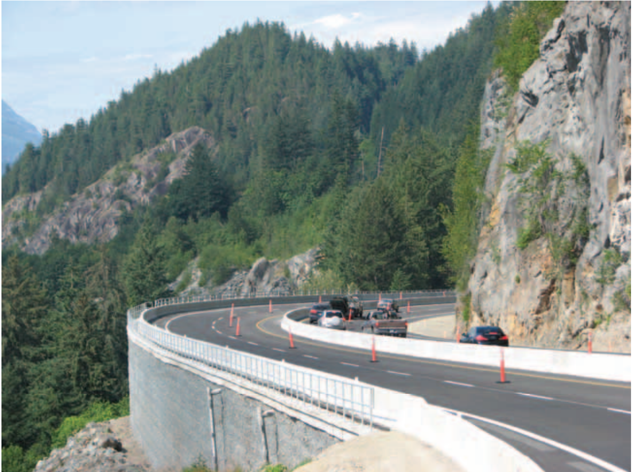
Completed section of Sea-to-Sky Highway, approximately 19 kilometres north of Horseshoe Bay, showing use of mechanically stabilized earth walls used to expand the highway on the down slope side of the highway.
